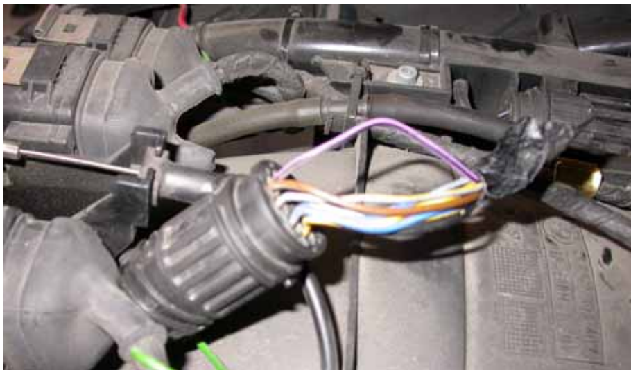
Figure 13. Purple wire for making "hot" connection
