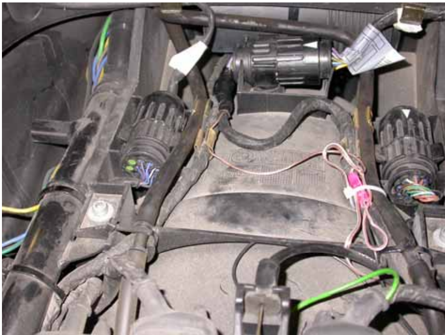
Figure 21. Wires routed and secured with cable tie for one light (viewed looking back from driver's seat)
