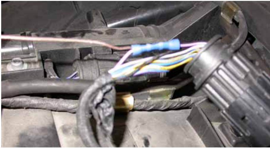
Figure 15. Blue butt connector attached to wires
